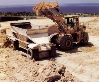
Above: These luxury view project sites in south Orange County are a specialty of Greg Kuno. He has developed a special expertise in coping with the size, multi-level excavations, and frequent change orders required by the owner, the architect, planners, soils technicians and regulatory agencies. This particular lot covers an estimated five acres.
